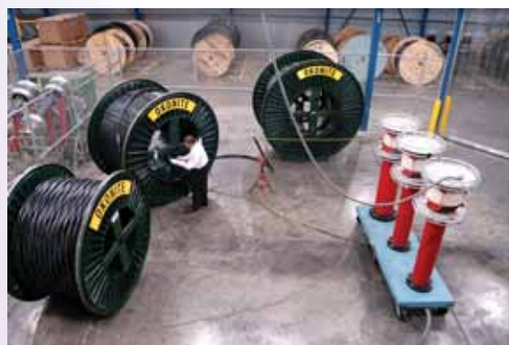
Voltage tests completed on three reels.
