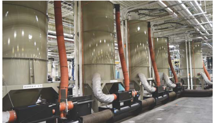
Central drying system for the insulating department. Dedicated dryer hoppers allow for materials to be pre-dried and isolated, allowing for rapid product changes.
